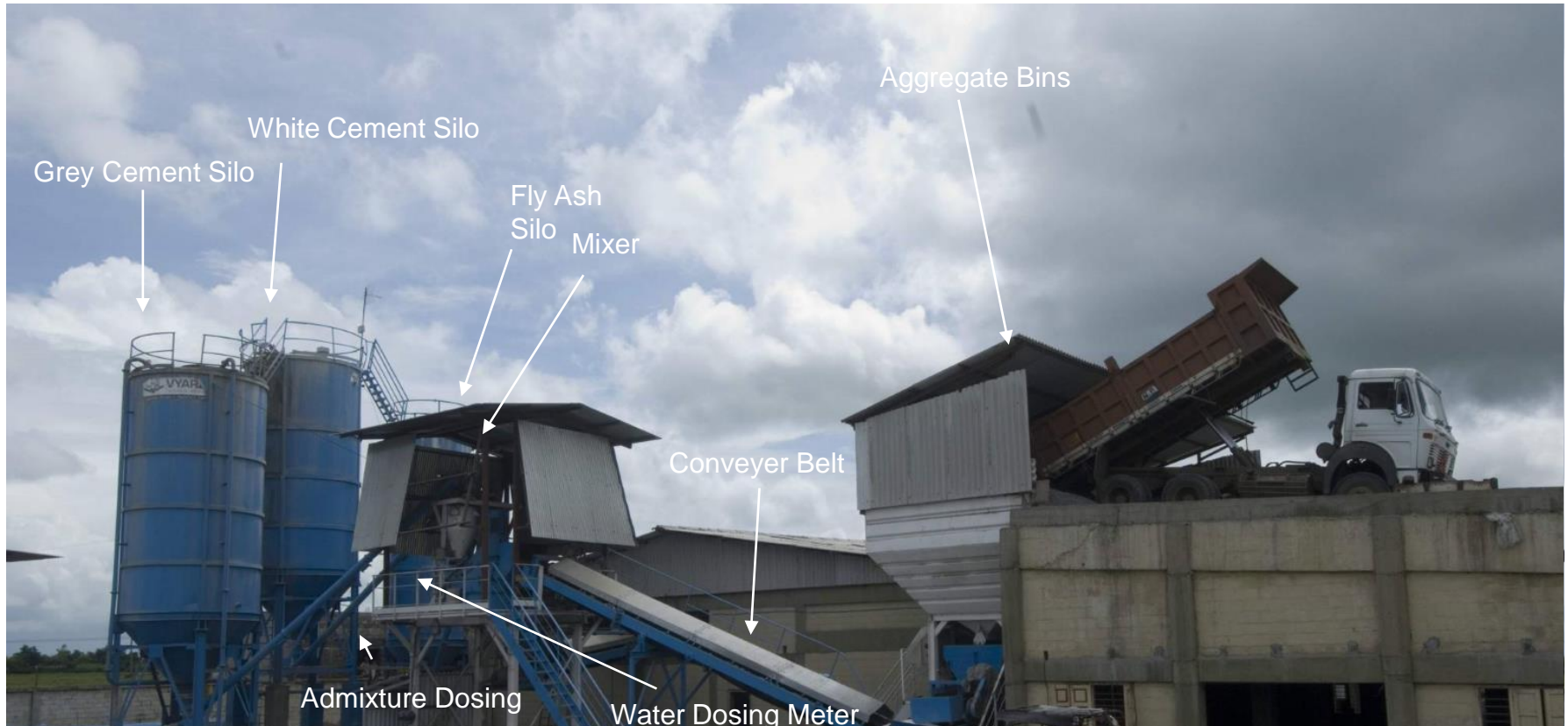
Fully Automatic Computerized Weigh Batching Plant and Mixing Plant
