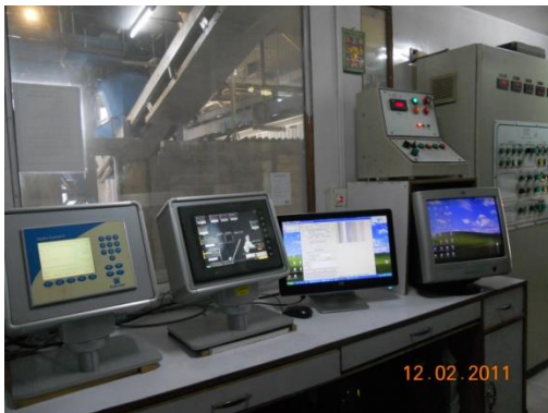
Moisture control in Bins and Mixer
